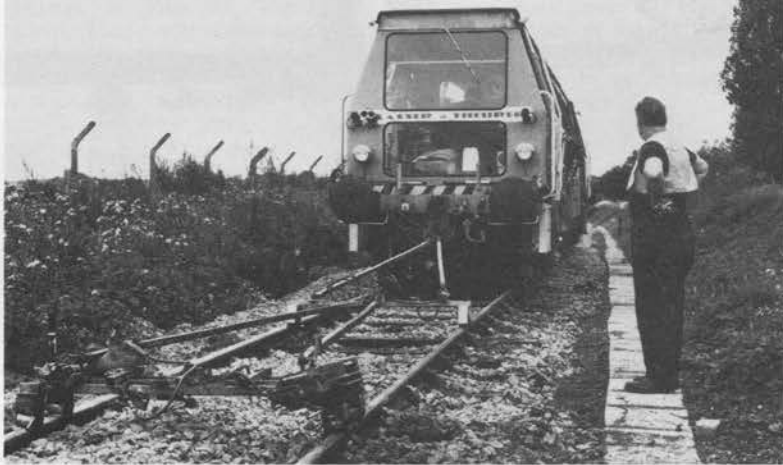
Top quality alignment and firmness resulted on the Main Line extension from a visit by a BR tamping/lining machine in August 1986, seen here next to the foundation of the new station platform.
