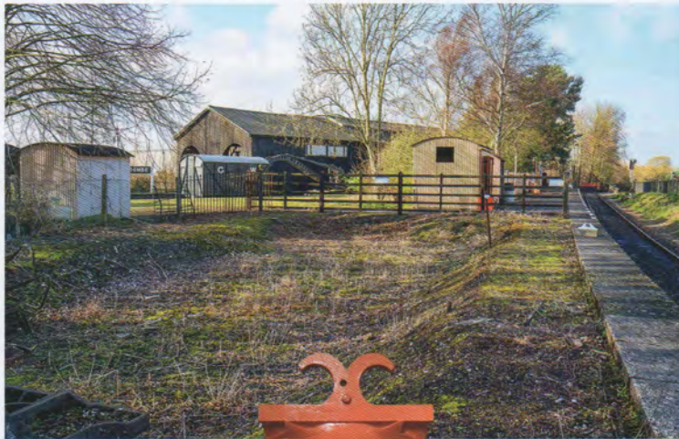
Below: The site at Oxford Road for reconstruction of the Heyford building has been prepared for the foundation slab, seen on 12 March 2020. An early benefit of the scheme will be to bring the adjacent section of the Oxford Road platform into use for visitors. Frank Dumbleton
